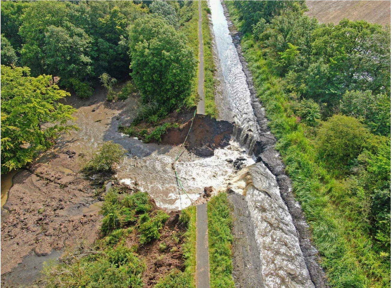
Figure 6: Breach of the Union Canal resulting in water from the canal to spread across neighbouring fields and flooded the Edinburgh to Glasgow rail line. Source: Scottish Canals ( www.scottishcanals.co.uk ).
